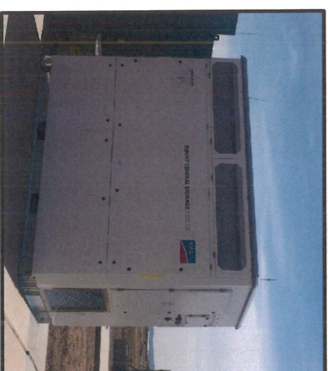
Pad-mounted Inverter (DC to AC)
