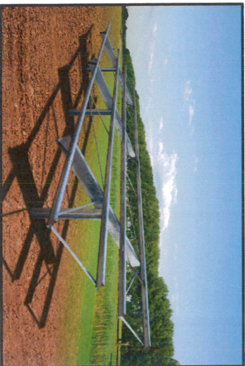
Solar Racking on driven posts
