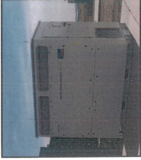
Pad-mounted Inverter (DC to AC)
