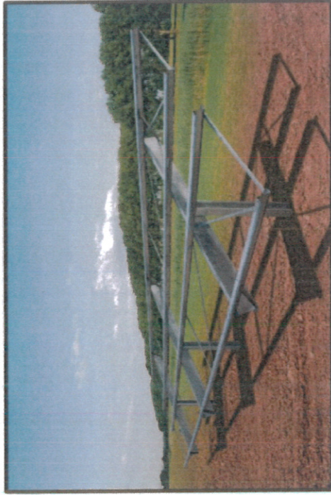
Solar Racking on driven posts
